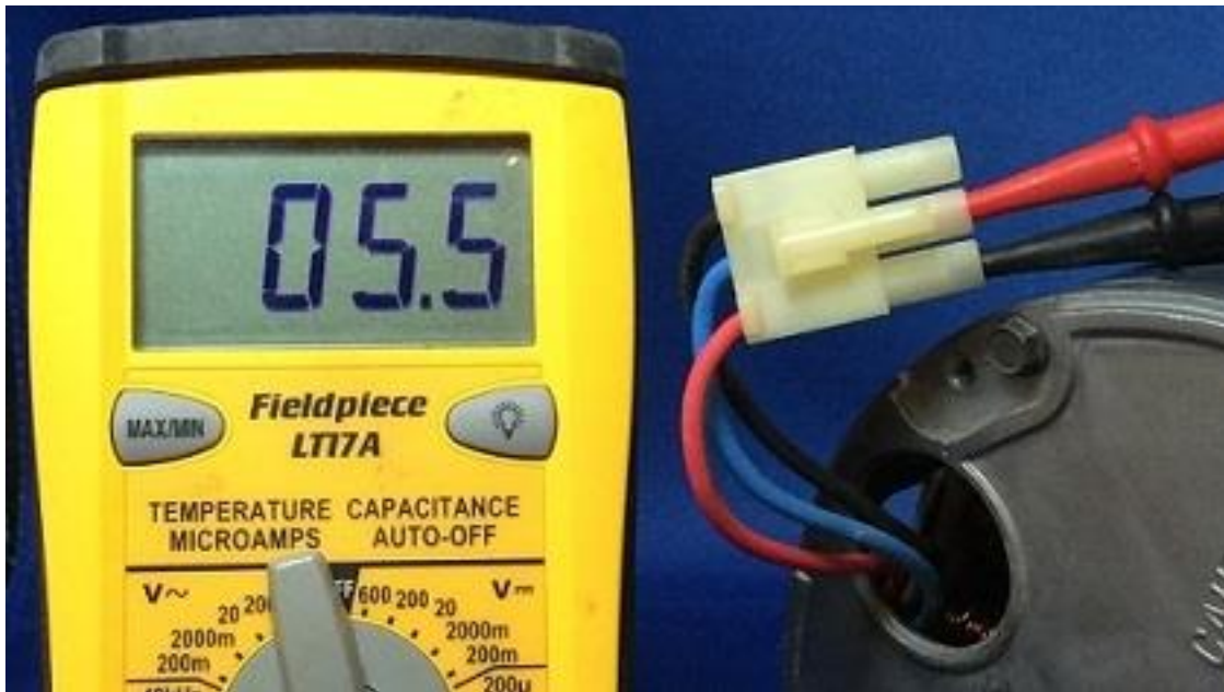
Figure 7-76 With a test instrument set properly, the windings of an ECM motor can be checked for resistance. Here our meter shows 5.5 Ω.
