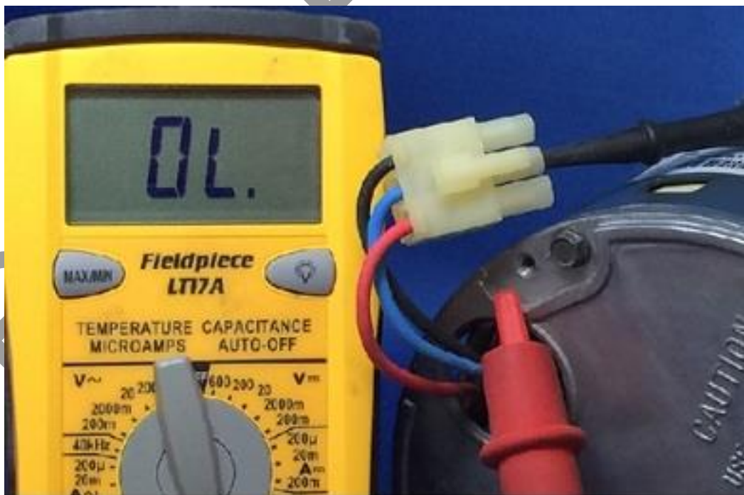
Figure 7-77 This test from a motor lead to the motor case shows that the motor winding is not shorted to ground. If the motor was grounded, the meter would show continuity.
