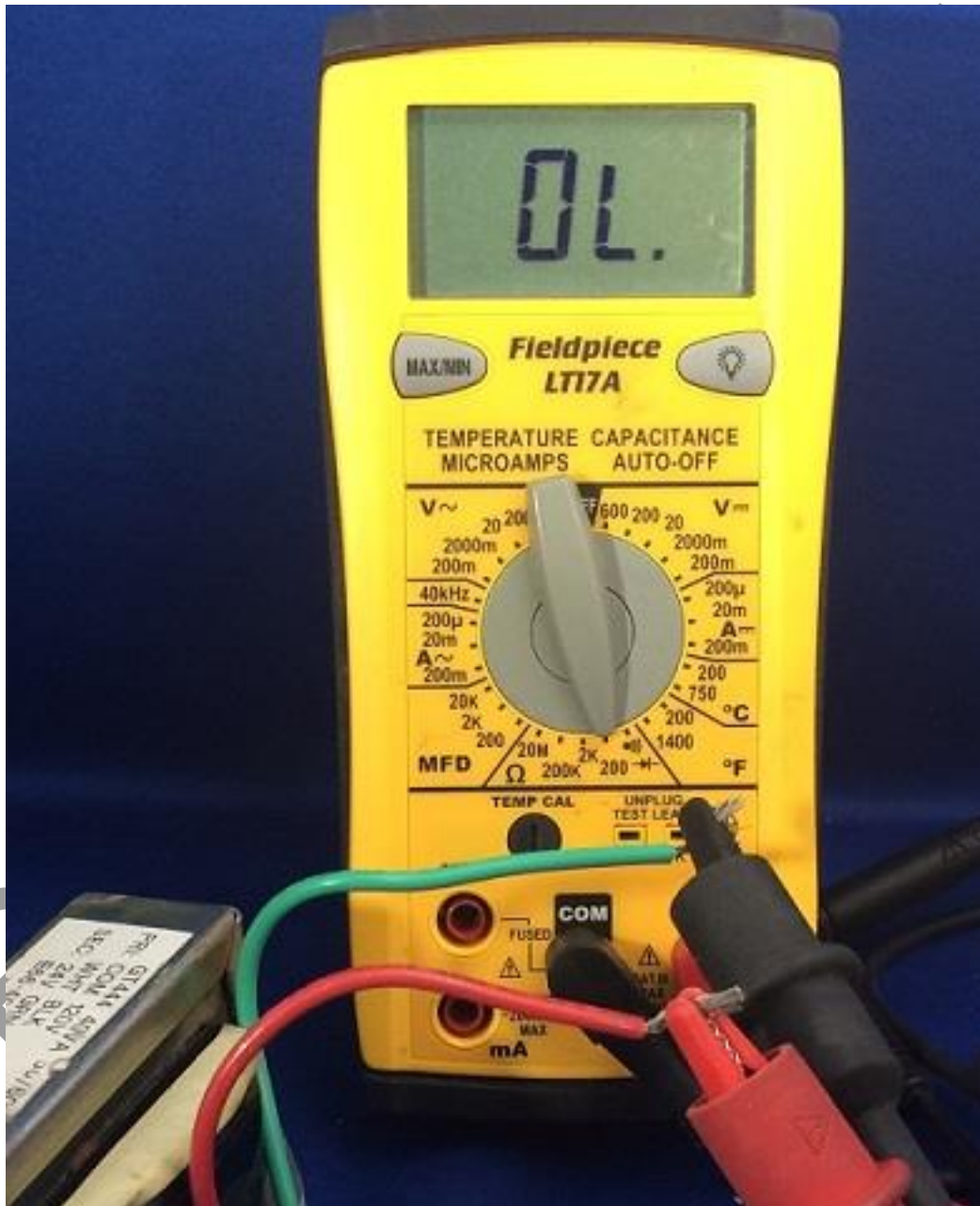
Figure 6-9 The secondary winding of this transformer has failed. The meter display is showing “OL” which is an indicator of “Open Line”.
