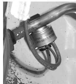
The TDL shown here is used to shut the heater off when the discharge line reaches a specific temperature during compressor operation.
