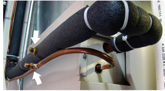
The indicated ports are about one foot in distance from the evaporator coil and metering device as noted above.
