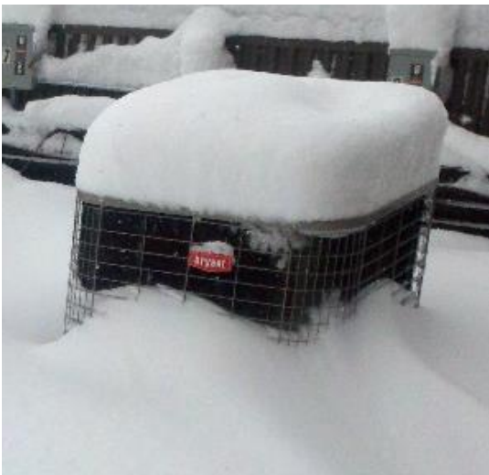
Figure 7-1 Residential equipment installed in a commercial environment will many times require operation in the winter.
