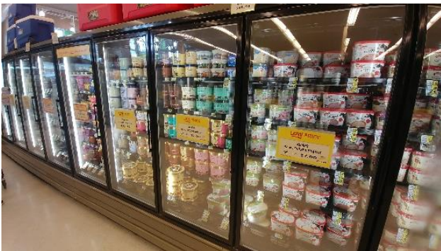
Figure 7-10 Grocery store freezer and refrigerator display case doors and door jambs are heated to prevent icing and fogging.
