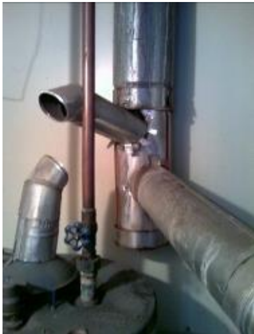
Figure 1-16 The single-wall water heater flue pipe broke apart at the seam, venting flue gas into the mechanical room.
