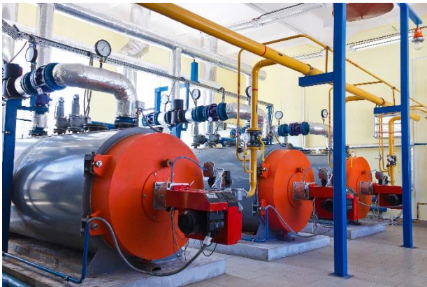
Figure 7-18 Commercial boilers are typically millions of BTUs with thousands of gallons of water involved. The initial heating process takes time and building switch-over from cooling to heating puts stress on the equipment.
