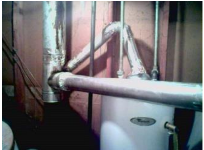
Figure 1-17 The entire flue stack fell over 3 feet from a faulty installation. Although creative, the re-connection of the water heater was completely illegal.
