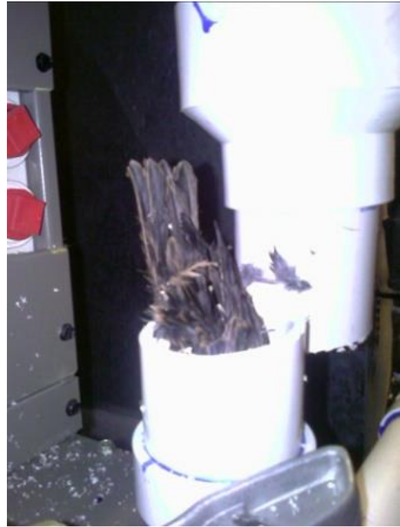
Figure 6-64 A bird in the flue at the inducer fan motor.
