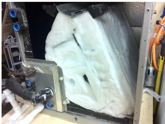
Figure 6-33 Ice on an evaporator can be many inches in thickness. The tell-tale sign (other than the obvious “hot house”) is that the blower is running but no air is coming out the registers. This coil would take at least 12 hours to thaw using the “fan-on” function, or a few minutes using a space heater directly onto the coil.
