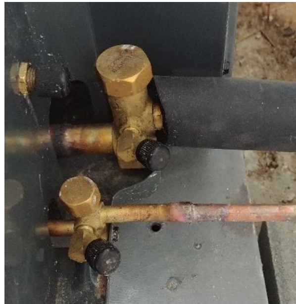
Figure 5-1 King Valves with service ports on a condenser where the line sets attach.
