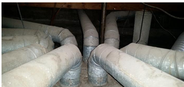
Figure 9-16 Bad ductwork can doom an otherwise good equipment installation. In this case, each duct is only 4 inches, there are too many separate runs, and none are insulated. Half of the capacity of the furnace was lost due to poor duct installation. Duct pressure is measured in Inches of Water Column.
