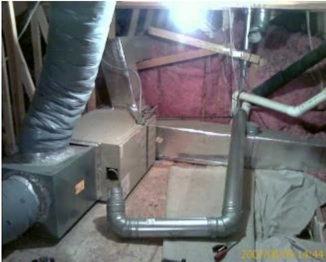
Figure 1-15 A 12-foot section of unsupported flue pipe became dislodged, venting flue gas directly into the attic.
