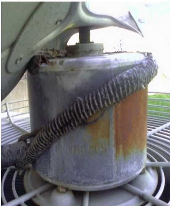
Figure 6-63 A snake burned out a condenser fan motor.
