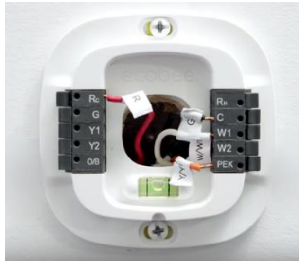
Figure 3-9 Where thermostat wires are attached to the base tell the smart thermostat what equipment is installed. The thermostat must then be programmed to refine the equipment selection (gas or electric heat, when to switch between multiple stages of heat / cool, what type of heat pump is installed, balance point, dead zone, etc.).
